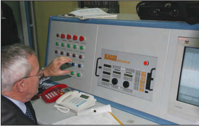
China Gas Turbine Establishment control room with the Kahn Series 545 control console installed.
